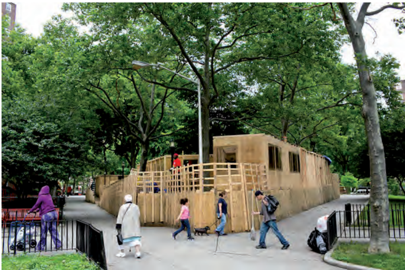
The temporary Gramsci Monument, under construction at the Forest Houses development in the South Bronx
